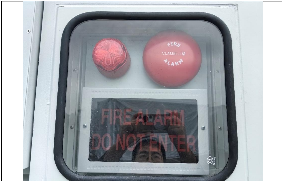
External fire alarm panel with protection
