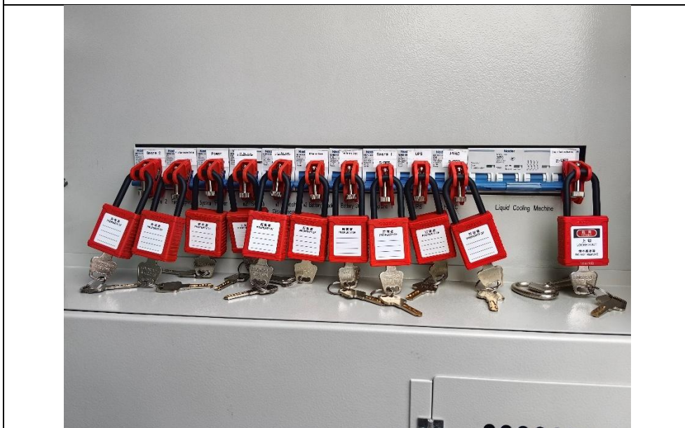
AUX power cabinet switch with locking method
