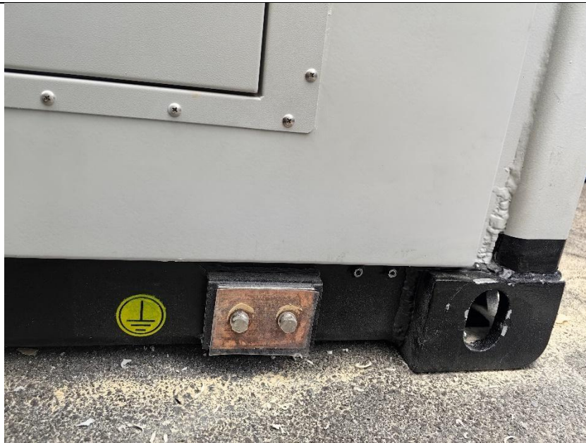
Container earthing terminal
