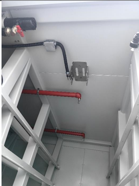
Water fire protection
